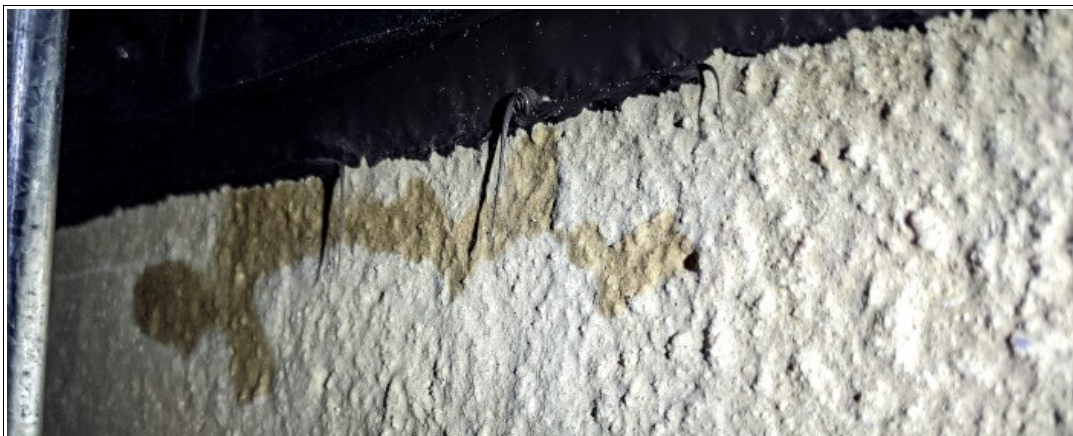
Otherwise Imperceptible Cracks in Substrate - Missed if Test Chamber Isolation & Observation Excludes Substrate
